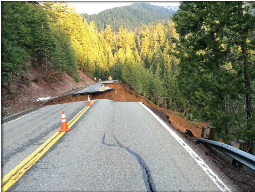
Slip-out of CA State Route 3 above Slate Creek, 2016. (Photo courtesy of Caltrans North Region Environmental Stewardship)
