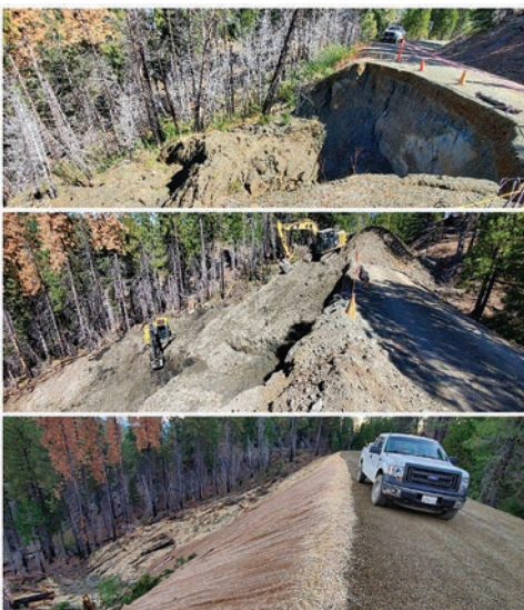
Before, during and after reconstruction on the Lassic Loop Road in the SRNF
