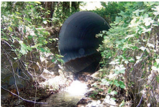
The culvert that will be replaced with an arched culvert at a USFS campground in Weaverville. (5 Counties Salmonid Conservation Program)
